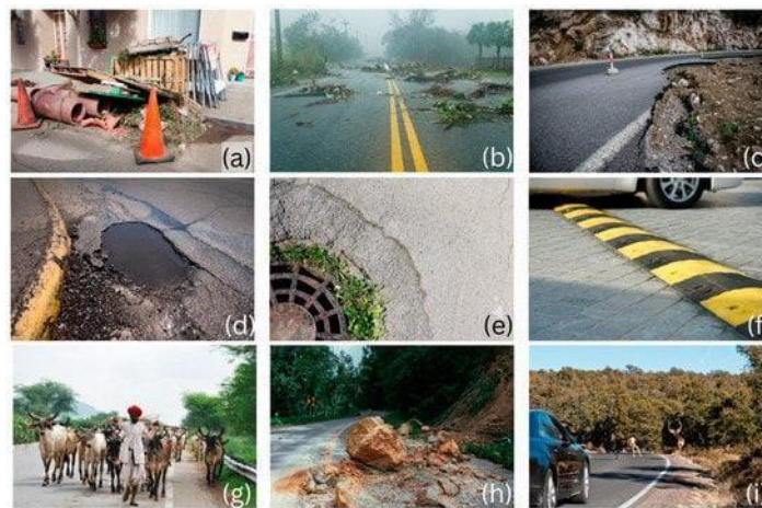
Figure 1: Various types of roadside anomalies and defects, including (a) road maintenance objects and construction debris, (b) debris fallen on-road, (c) road surface failure, (d) potholes, (e) maintenance holes and pseudo potholes, (f) speed bumps, (g) farm animals on the road, a common on-road hazard type, (h) landslide debris, and (i) wild animals jumping in front of a speeding car.
